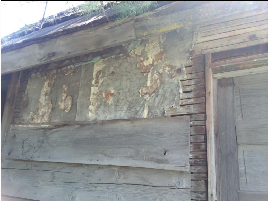
FIGURE 14: WESTERN OUTSIDE WALL SHOWING LATH AND MUSLIN BACKED WALLPAPER ON WHAT WAS AN INTERIOR WALL.
