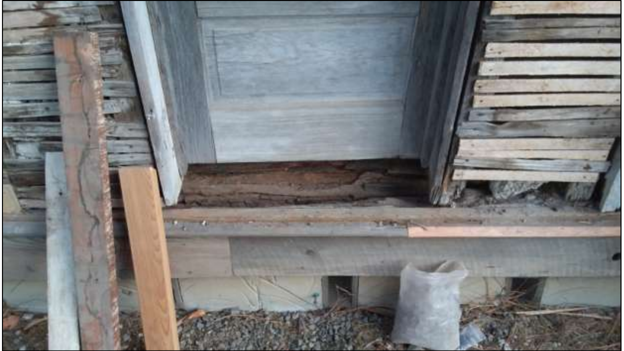
Figure 3. Sill rot in west doorway, beans found in this location.
